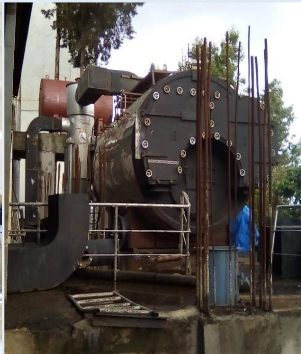
Newly installed Boiler at Uplands dairies ltd
