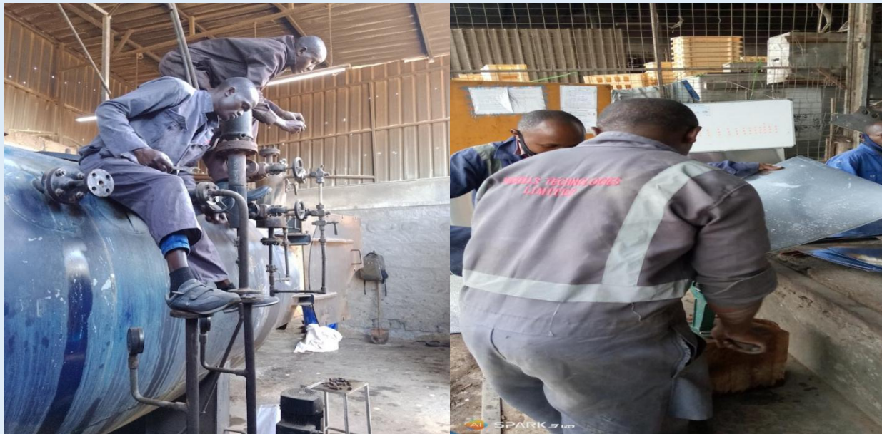
Boiler service at Devayni foods ltd (Daima Dairies)
